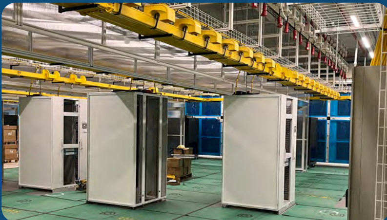
Brooklyn data center
